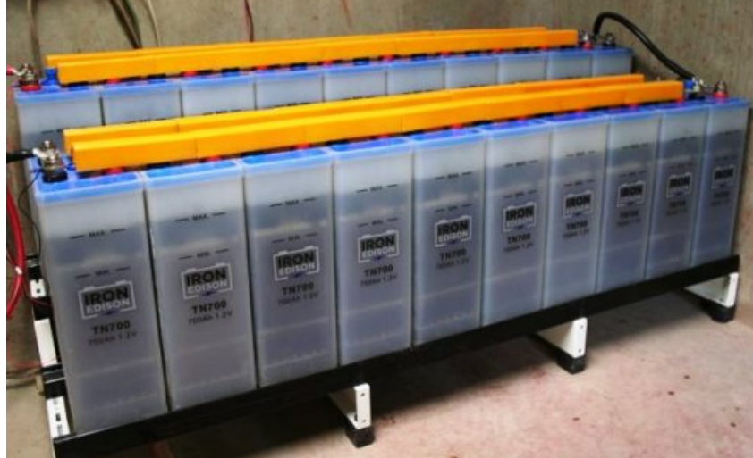
Figure 7.3.2 Iron Edison Nickel Iron Battery Bank
